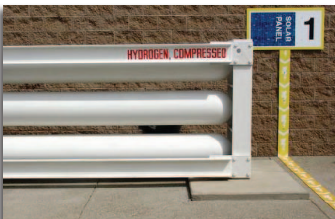
Compressed hydrogen storage tanks at the SMUD solar-powered hydrogen vehicle fueling station in Sacramento, California.
